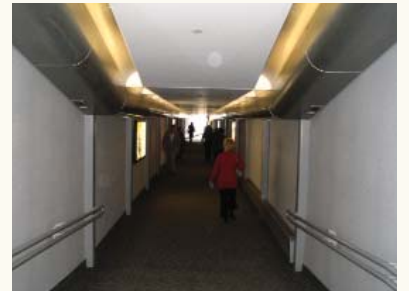
Updates to the skyway transformed it from a dark tunnel (above) to a bright and welcoming portal.
